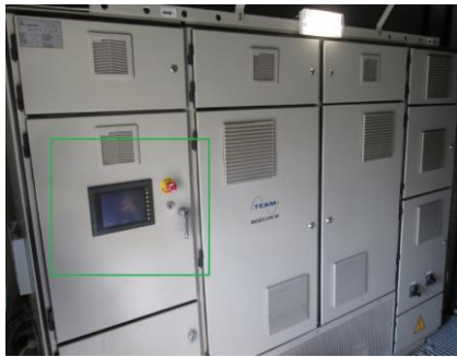
Armario ground, señalado en verde el panel de control. Ground cabinet with the control panel outlined in green.
